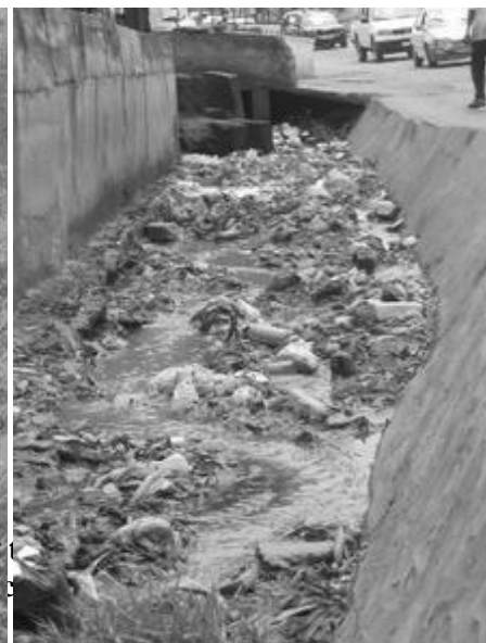
Figure 14: Clogged gutter in Accra
