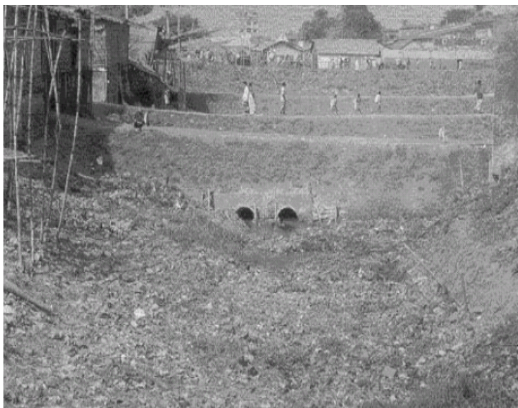
Figure 13: Clogging of city drains due to solid waste dumping in Dhaka [24]
